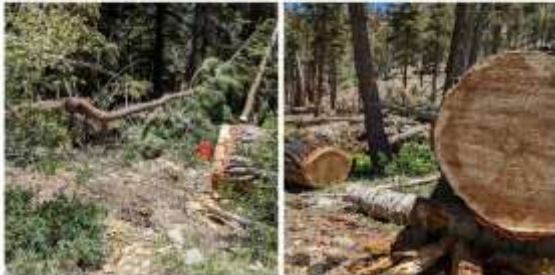
South Fork Trail is passable again after our trail crew spent several days clearing dozens of fallen trees and avalanche debris. Photos by Nelva Valladares
