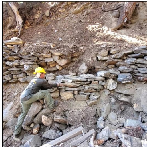
Trail boss David Bratt helps rebuild a rock wall on the Falls Creek Trail in August. Photo by Nelva Valladares
